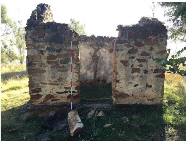
Plate 62. South entrance with collapsed lintel of outbuilding (North)
