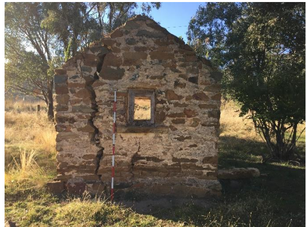
Plate 61. West wall with window and a large crack running the height of the wall of outbuilding (East)
