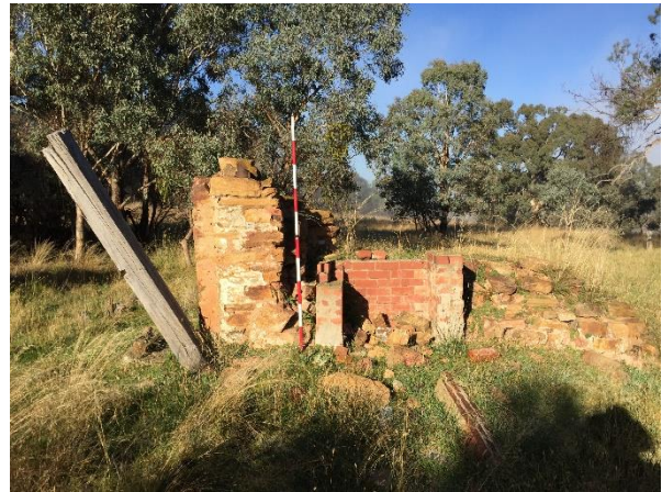
Plate 59. Timber support post leaning East, with partial stone wall and fireplace (South)
